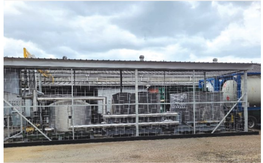
Batch Chiller Facility
